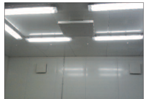
Typical passive laser safety enclosure
